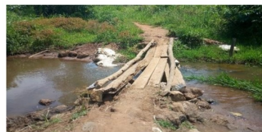
First picture: Condition of the former makeshift ARILE bridge. View of the layers of dead wood and planks used to secure passage.
